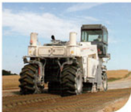
A1 road bits for the A1: all of the machines on Europe's largest road construction site are fitted with Betek road construction tools.
